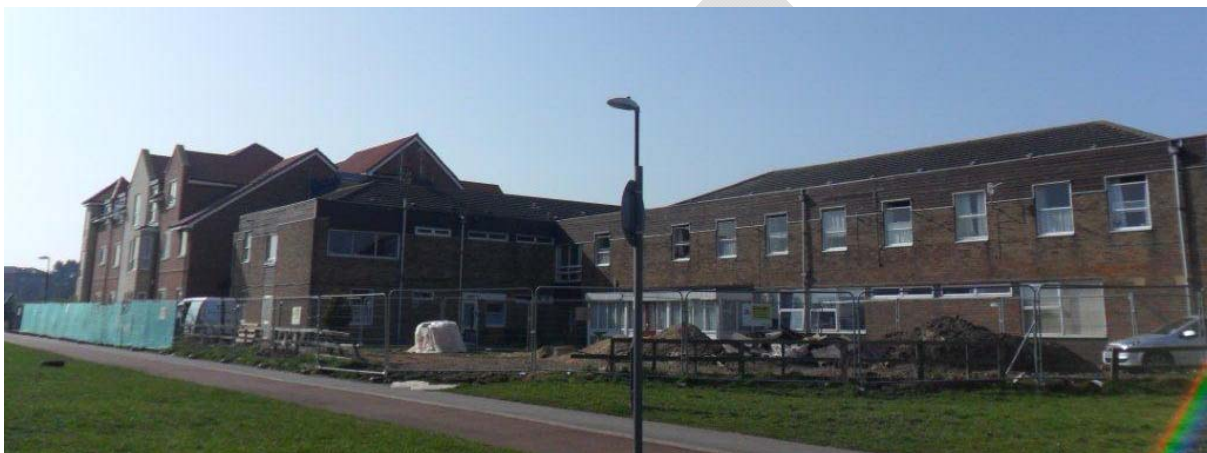
Cherry Garth Elderly Persons' Home transforming in a two-phase build process into Meadowfields Extra Care
